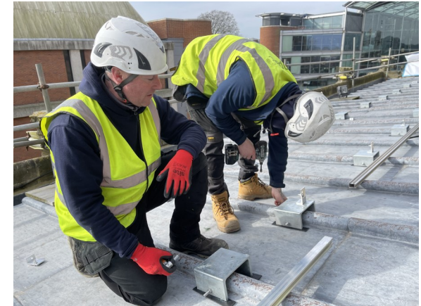
Contractors from local business Impact Services preparing the South aisle roof for the solar panels
